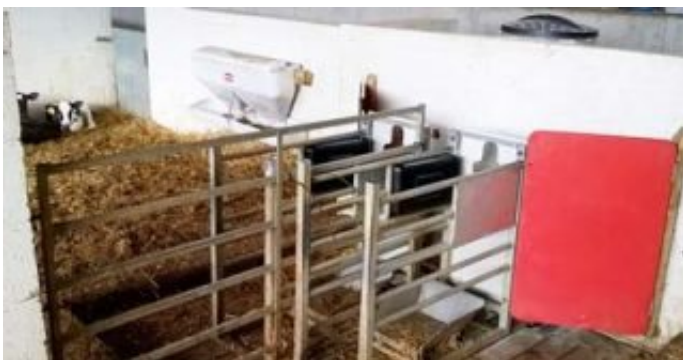
Figure 7. Automatic feeding areas can be focal zones for the buildup of moisture and pathogens.
