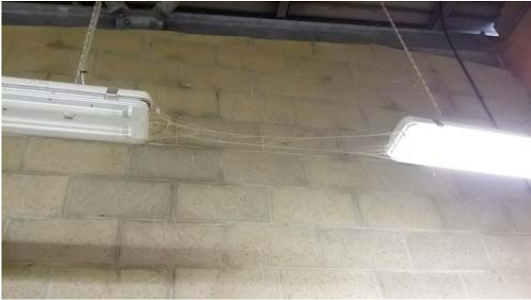
Figure 6. The presence of cobwebs can be a visual indicator of poor airflow through a building.
